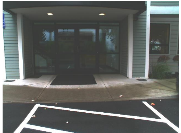
Curb Ramp : No Detectable Warnings
