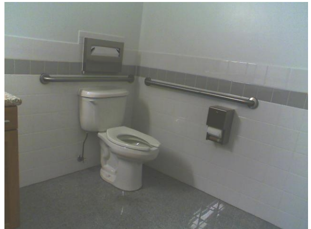
Restroom , Toilet : Toilet Distance From Wall
