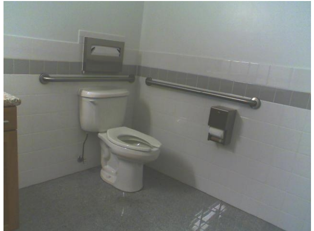
Restroom , Toilet Compartment : Toilet Paper Dispenser Distance From Seat
